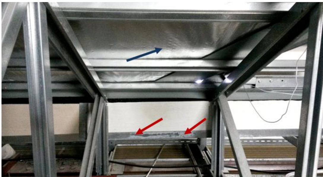
Fig. 10. Localized white rust (corrosion) was observed on the galvanized steel bar channels (red arrows) and the insulation attached to the underside of the roof (blue arrows)
